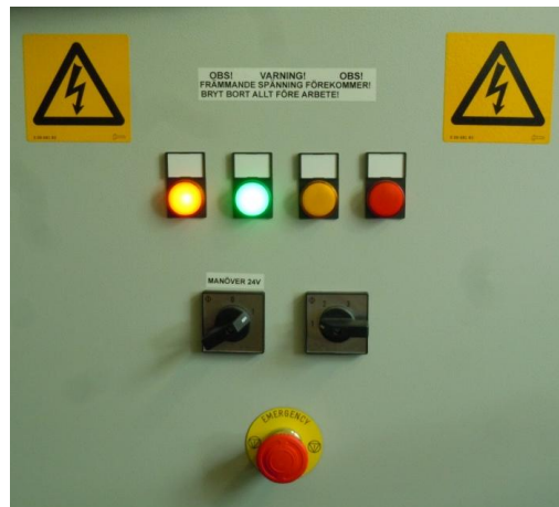
Figure 43 - Notification lights on the grid side cabinet
