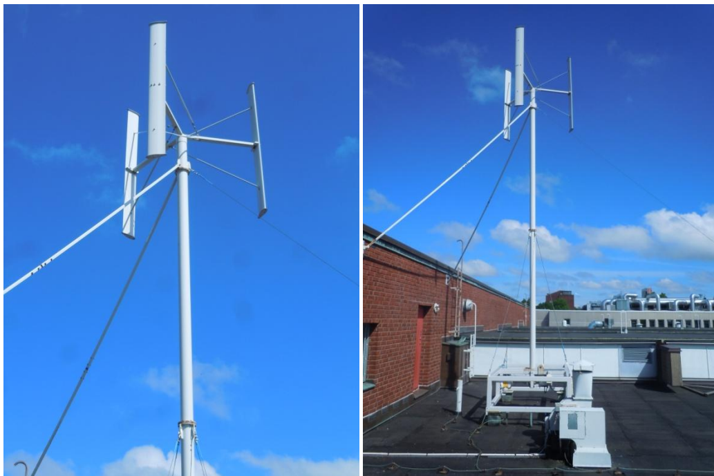
Figure 22 - Wind turbine installation on the rooftop
